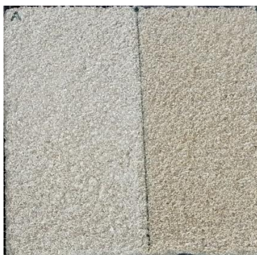
Hydrophobic capacity of the Puerto stone. Given its high porosity, no pearl effect occurs, but it can be seen how the untreated area is darker due to the absorption of water compared to the treated area.
